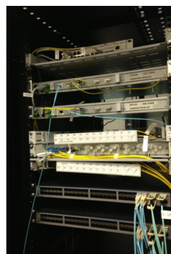
VBM Equipment in Rack
